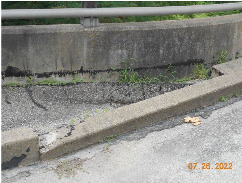
Existing Approach Slab Settlement
