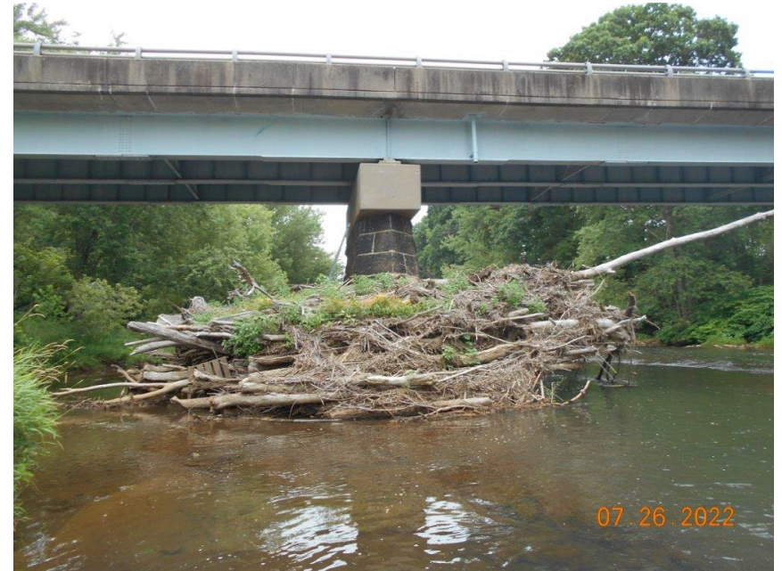
Existing Debris Build-up
