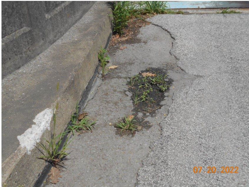
Existing Approach Slab Settlement
