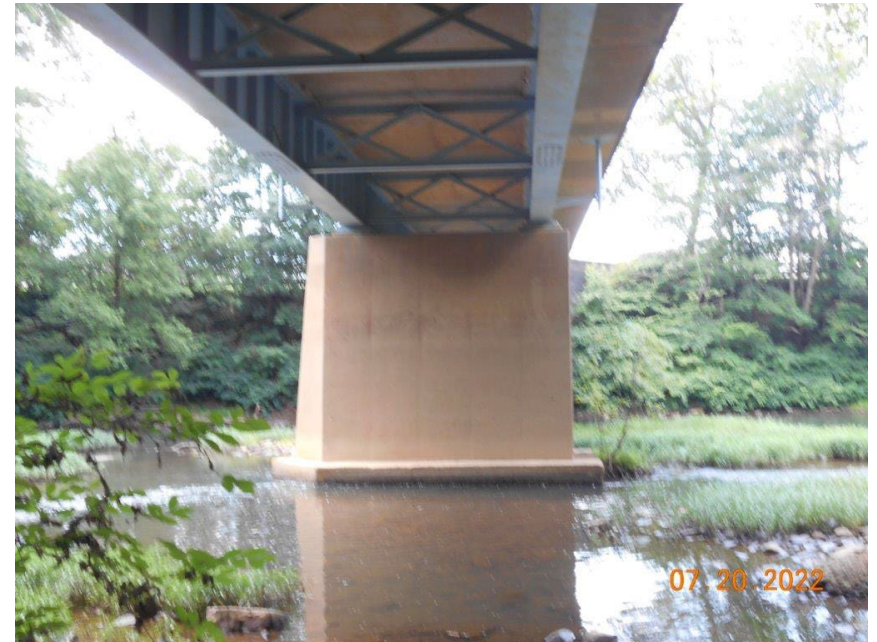
Existing Debris Build-up
