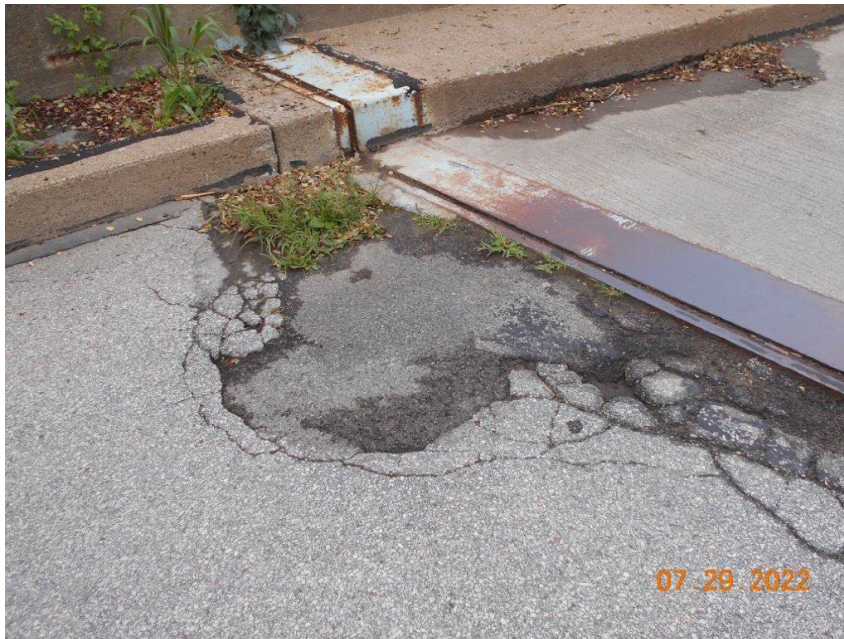
Existing Approach Slab Settlement
