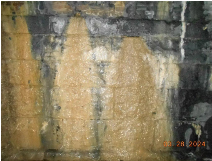
Leaking at Mortar Loss
