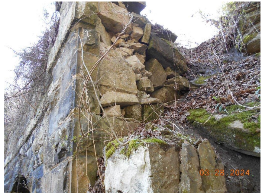
Erosion at Portal
