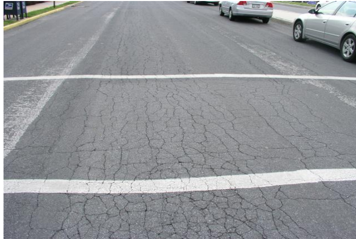
Photo 12, Condition of road prior to placement of product.
