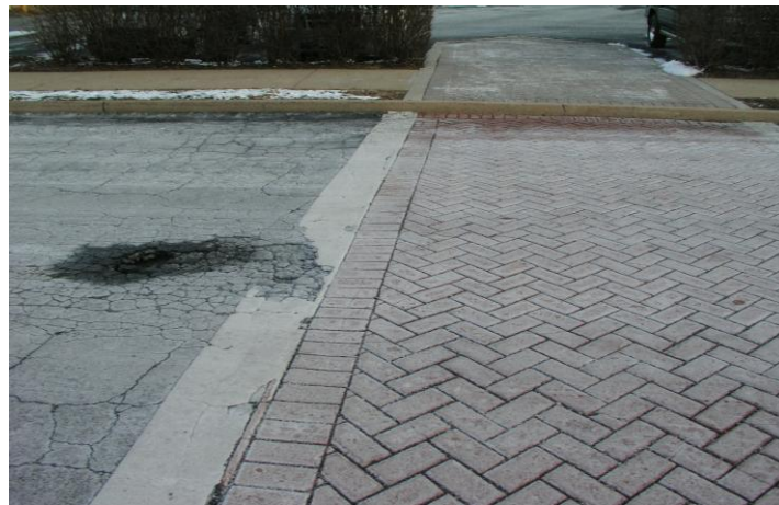
Photo 13, Additional deterioration of road after placement.
